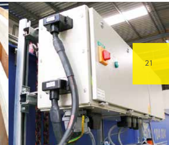
Bridge panel with plugs
