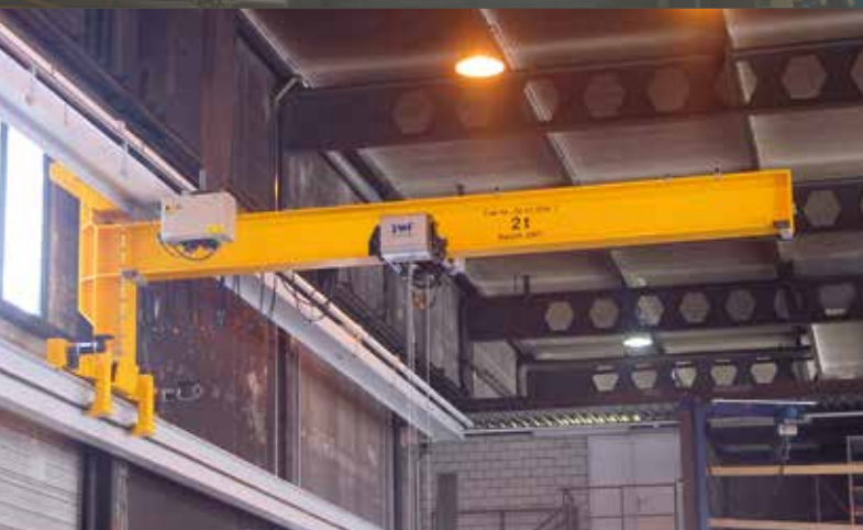
Wall console crane
