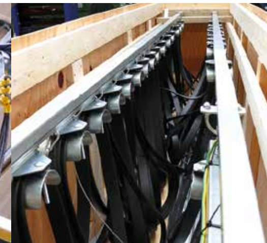
Ready to use hoist power supply
